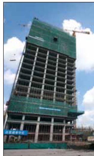
Construction site of the AIA's Asia-Pacific finance center, in the Guangdong High-Tech Service Zone of Financial Institutions.
